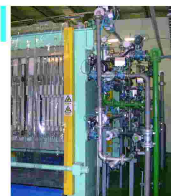
PLC控制所有阀门 All valves are controlled by PLC
