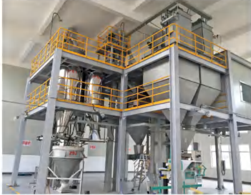
自动配料包装生产线 Automatic batching and packing production line
