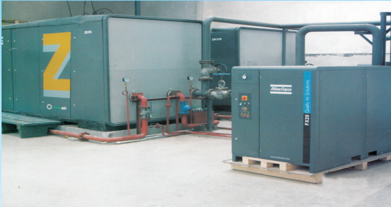
空压机/Atlas Oil Free Compressor
